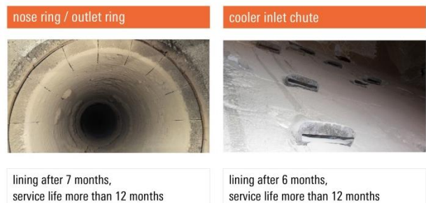
Fig. 7: Cement-free geopolymer bonded bauxite concrete in highly loaded areas of cement plants
